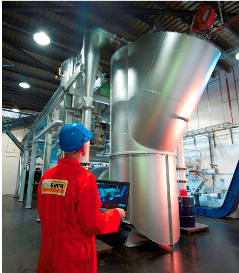
Advanced Thermal Unit, image courtesy of New Earth Solutions
